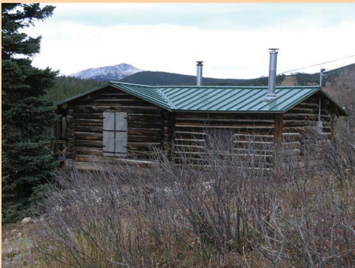
The historic Haffner cabin with its new green metal roof has a breathtaking view of Peterson Lake and James Peak.
