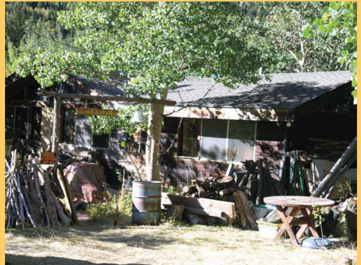
Cheerio Cabin at 844 Klondyke suffered extensive fire, smoke and water damage Labor Day, September 6, 2010.
