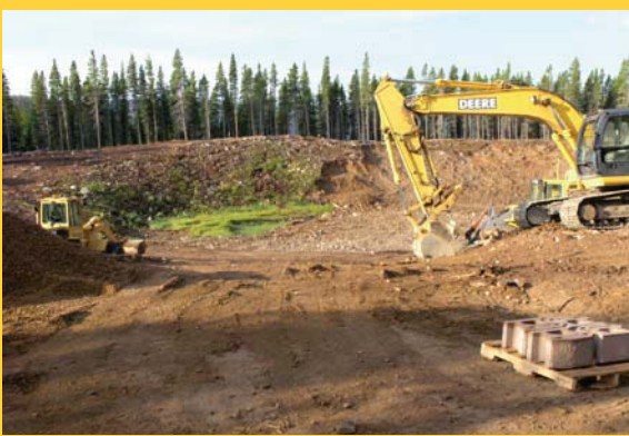
Heavy machinery filled the kettle pond and widened the depression as a water storage reservoir for snowmaking.
